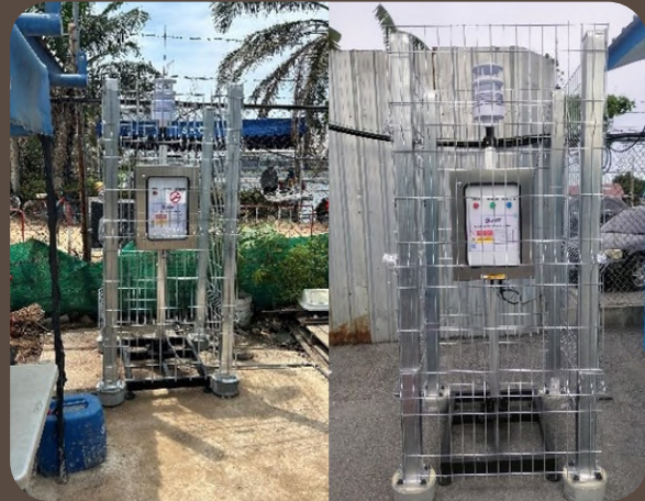
Experimental installation of the E-Nose system in the Thaioil Group area.
